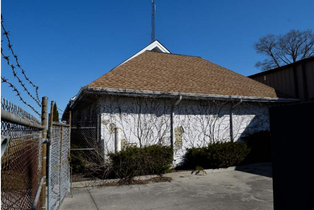
FIGURE 14: SOUTH FACE, FACING NORTH, NOTE THE EXPOSED YELLOW BRICK WHERE WHITE PAINT HAS EXFOLIATED
