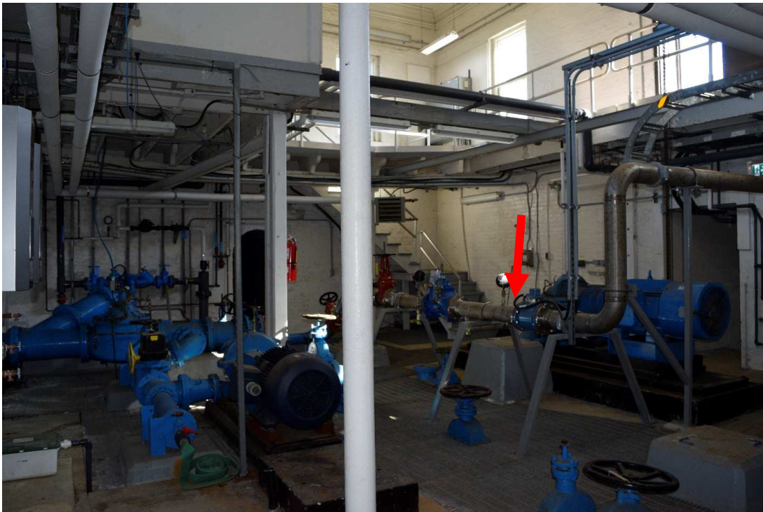
FIGURE 2: BELOW GRADE EGRESS OF WATER LINES WILL OCCUR IN THE GENERAL LOCATION OF ARROW
