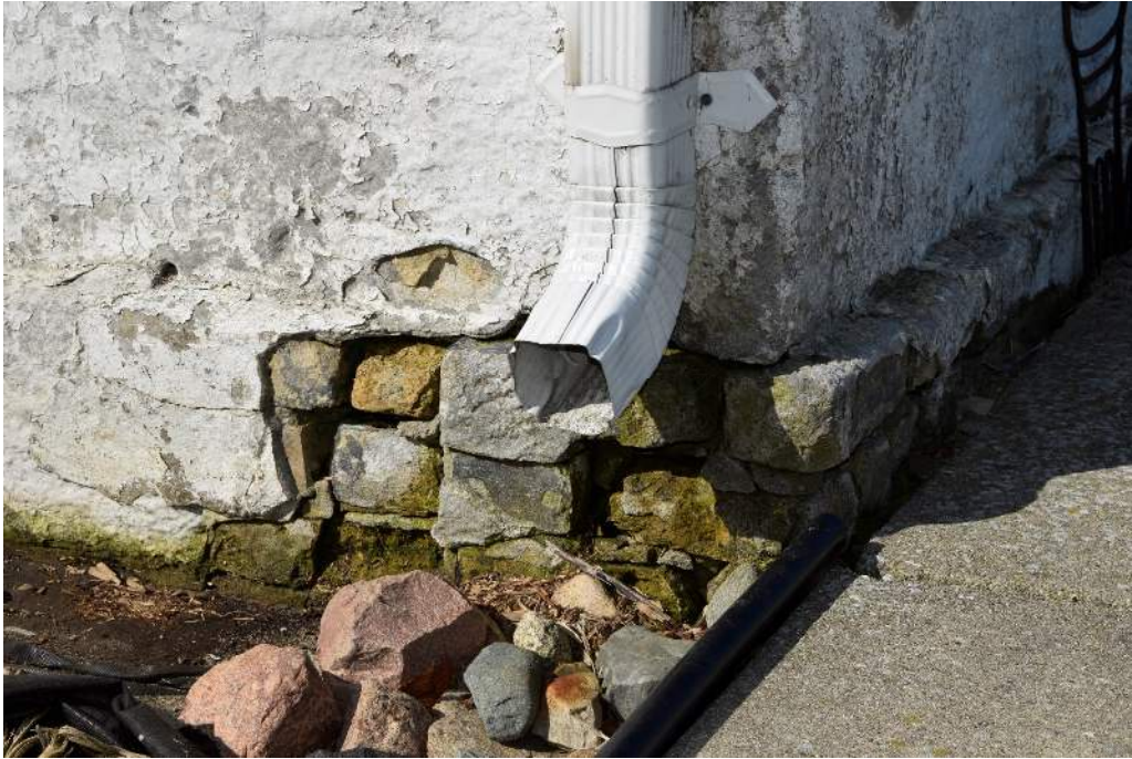
FIGURE 25: TYPICAL EXAMPLE OF DEGRADATION RESULTING FROM LACK OF WATER MANAGEMENT, EXPOSED YELLOW BRICK INDICATES STRUCTURE FOUNDATION IS OF SOFT YELLOW BRICK
