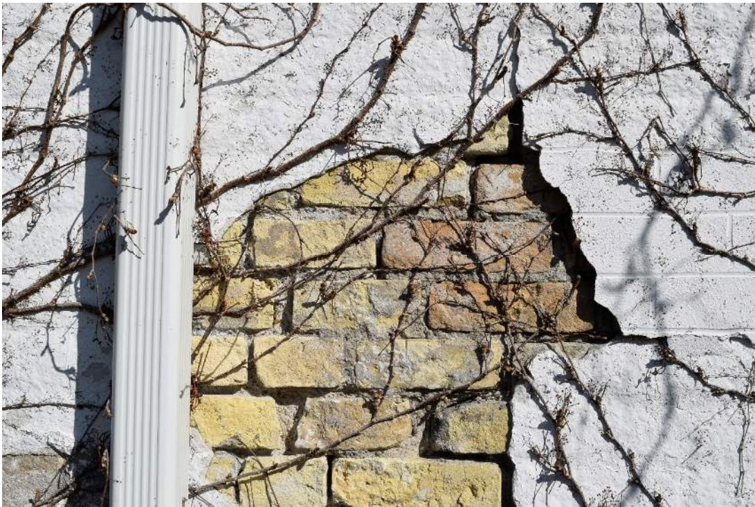
FIGURE 22: EXAMPLE OF EXFOLIATING PARGE COAT ON SOUTH SIDE OF STRUCTURE
