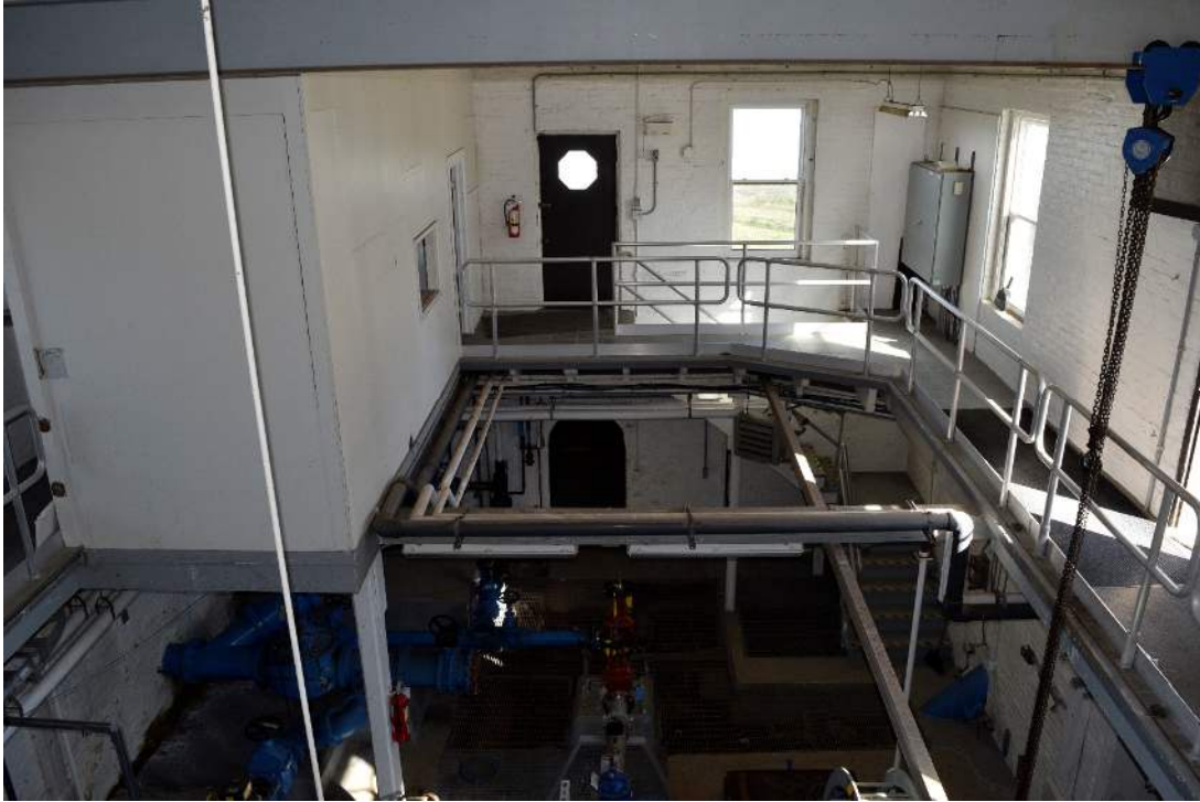
FIGURE 27: LOOKING NORTH FROM ELEVATED PLATFORM ON SOUTH END OF STRUCTURE, OFFICE IS ON LEFT OF IMAGE
