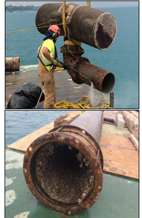
Photos taken of intake screen, pipe cut-out section, zebra mussel infestation, pipeline crack near the shoreline.
