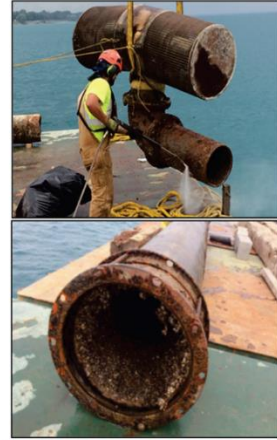
Photos taken of intake screen, pipe cut-out section, zebra mussel infestation, pipeline crack near the shoreline.
