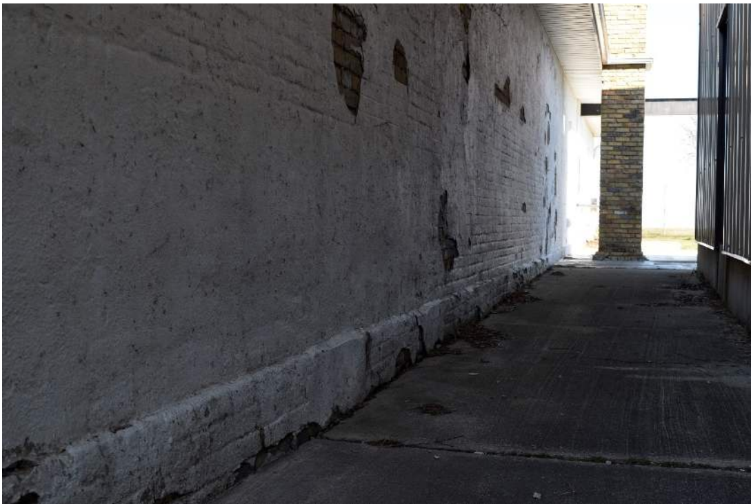
FIGURE 24: OVERALL CONDITION OF EAST SIDE OF STRUCTURE, FACING NORTH, NOTE REPEATED EXAMPLES OF PATCH WORK TO PARGE COAT AS EVIDENT BY DIFFERENT TEXTURES
