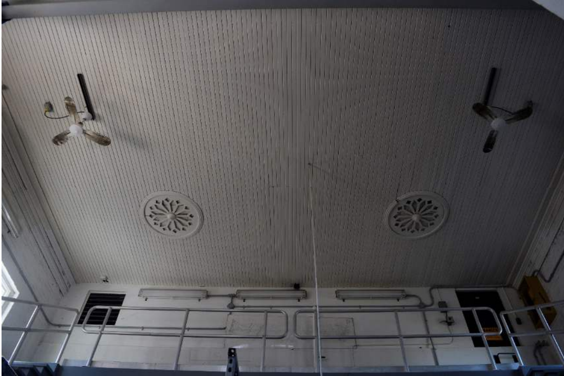
FIGURE 41: EXAMPLE OF ORIGINAL TONGUE AND GROOVE CEILING WITH DECORATIVE MEDALLIONS, SOUTH END OF STRUCTURE
