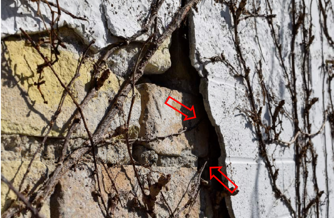
FIGURE 23: CLOSEUP OF THE SEPARATION OF PARGE COAT FROM UNDERLYING YELLOW BRICK, NOTE THE VINE RUNNER GROWING BETWEEN PARGE COAT AND YELLOW BRICK (RED ARROWS)
