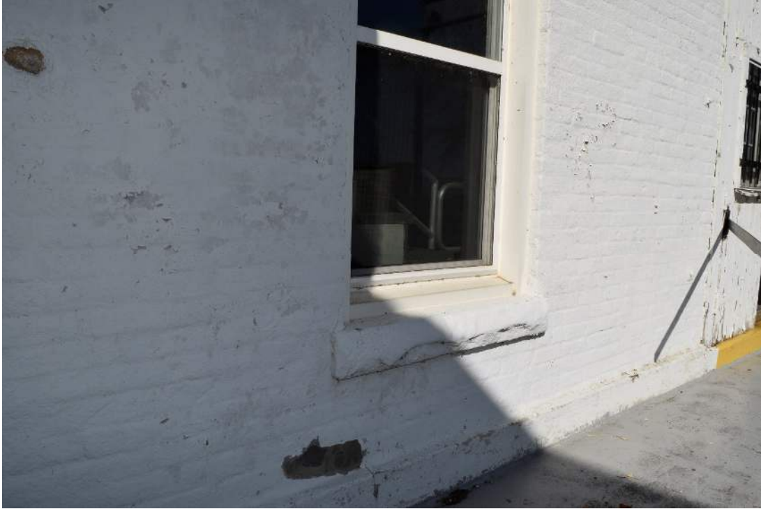
FIGURE 18: EXAMPLE OF TYPICAL CUT STONE LUG SILL, NOTE USE OF MODERN REPLACEMENT WINDOWS
