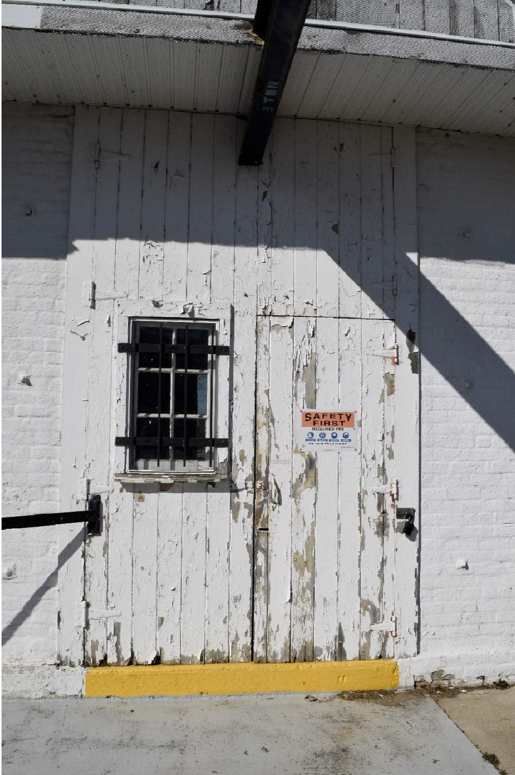
FIGURE 17: HEAVY EQUIPMENT EGRESS WITH INTEGRATED STANDARD EGRESS DOOR, LIKELY ADDED AS PART OF THE 1929 UPGRADES TO FACILITATE THE INCLUSION OF A CHLORINATION SYSTEM
