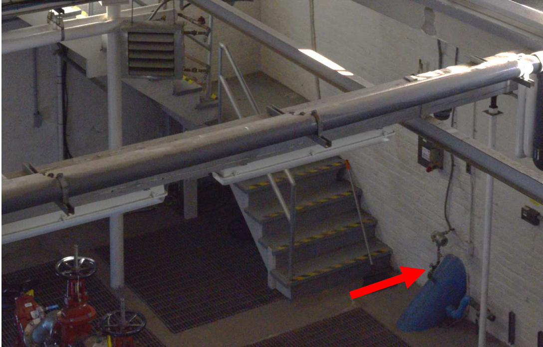
FIGURE 3: CLOSE UP OF EXISTING PIPING RUNNING THROUGH FOUNDATION IN SAME LOCATION PROPOSED ALTERATIONS
