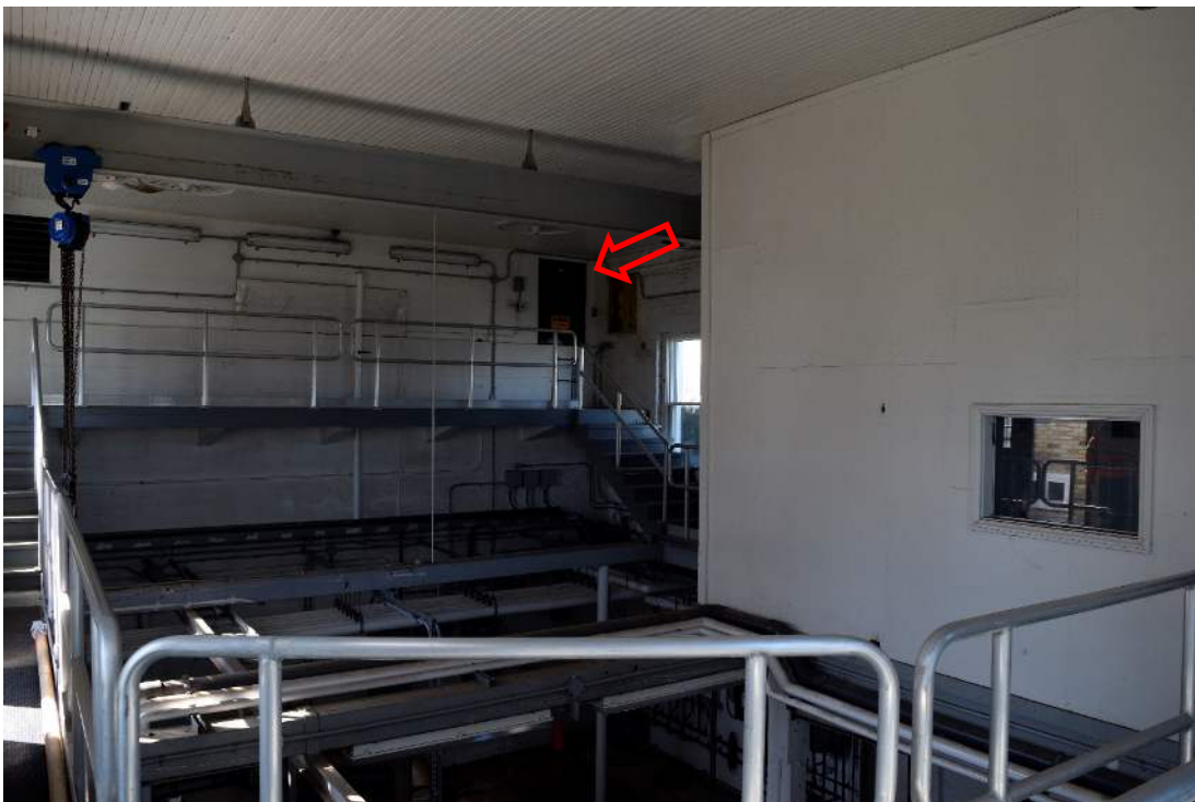
FIGURE 30: LOOKING SOUTH TOWARDS SOUTHWEST CORNER, RED ARROW INDICATED ACCESS HATCH TO ORIGINAL WATER SETTLING TANKS
