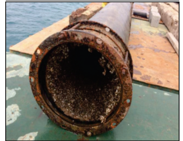
Photos taken of intake screen, pipe cut-out section, zebra mussel infestation, pipeline crack near the shoreline.
