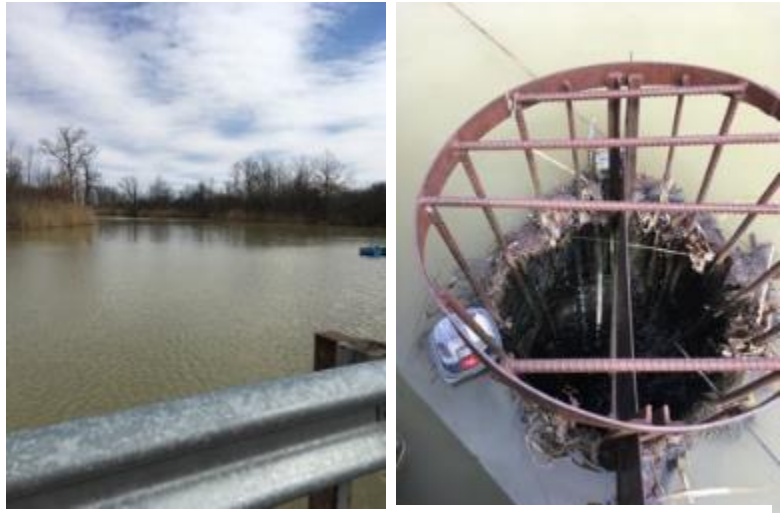
Existing Online Pond. Looking north from along retaining wall (left insert). Existing 600 mm CSP vertical pipe outlet (right insert).
